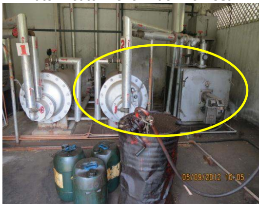
Gambar 6.12 Water Heater Boiler Machine Rosak
